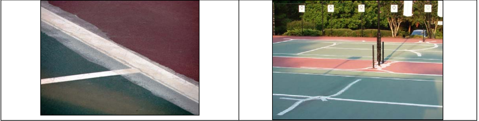
Dangerous cracks filled
